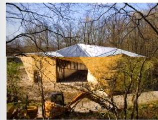
The faceted form is clad with western red cedar planking, sawn from trees felled on site.
